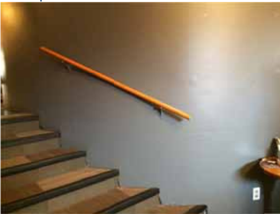
Figure 21: Handrail does not run the full length of staircase and does not level off at the top and bottom of the staircase.
