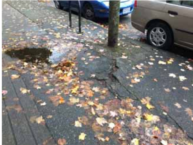
Figure 5: Cracked pavement, puddles and leaves on sidewalk in front of Firehall Arts Centre
