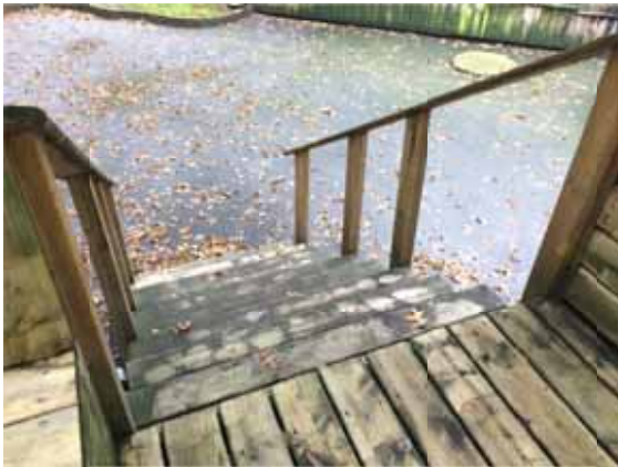
Figure 23: Stairs connecting outdoor patio area to rear courtyard lacks tactile warning strips & round handrails
