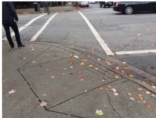
Figure 6: Example of a Curb ramp that does not line up with the accessible path of travel at intersection
