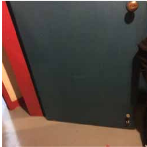
Figure 26: Washroom door with round handrail and without kick plate
